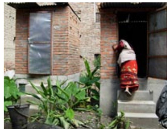
One of the 100 ecosan toilets, Photo: Dick de Jong, IRC
