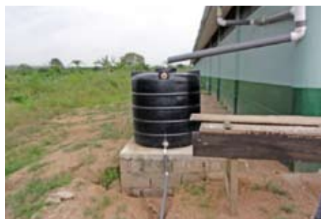
Water-tank to store rainfalls now used for flushing toilets and building all facilities. Photo: Caridad Machin Camacho, IRC.
