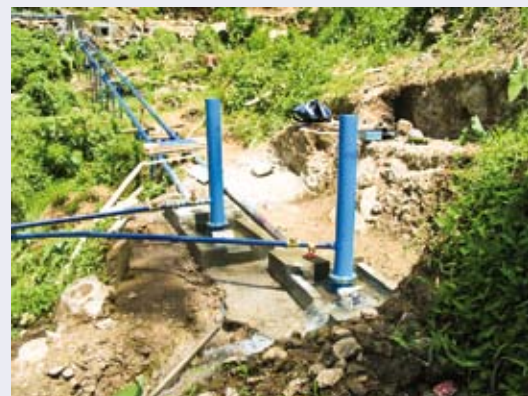
A typical Ram pump, see story starting p. 3
