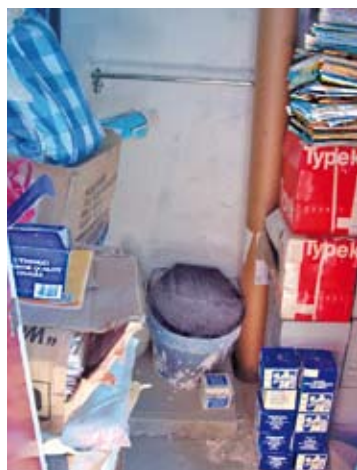
Toilet as storage. Photo: Dick de Jong, IRC
